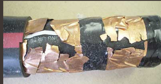
Crushed and broken cable shield
