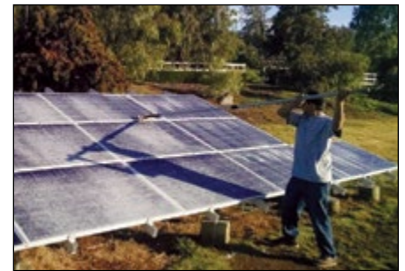
SPW™ being used to clean panels.
